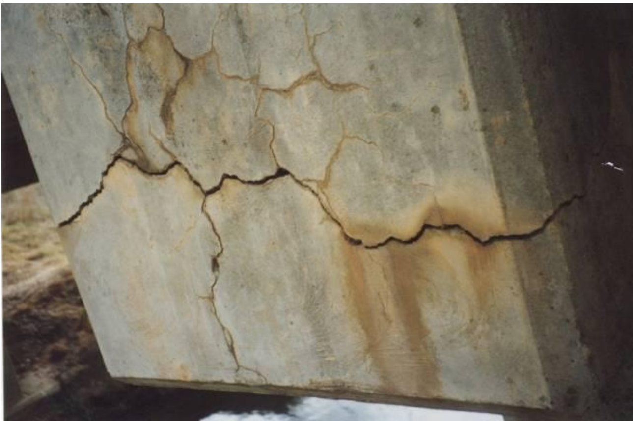
An Alkali Aggregate Reaction Cracked Bridge Element
